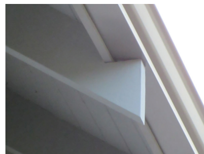
Fig. 1 Notched rafter ends
