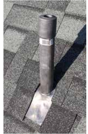
Fig. 3 Lead plumbing stack flashing
