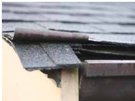
Fig. 6 Metal rain diverter directs water into gutter
