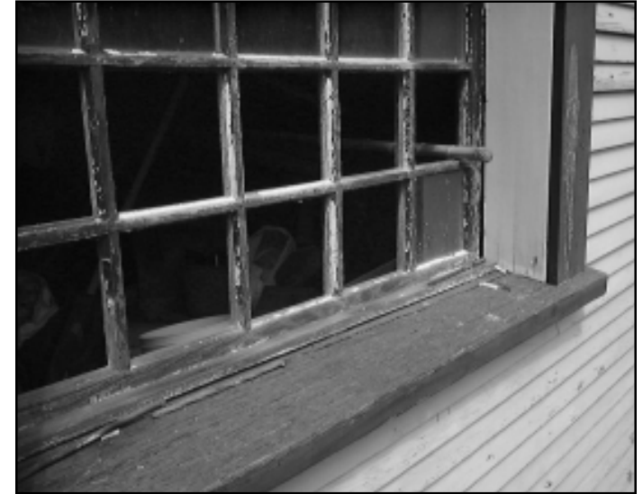
Damaged window sill
