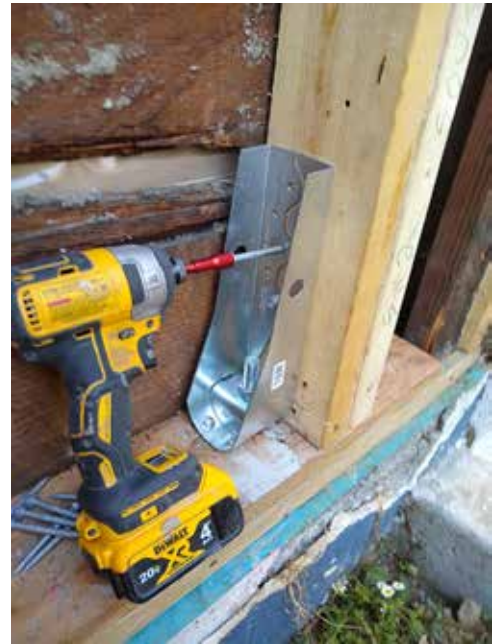
Hold-downs are installed at each end of all shear walls to resist uplift forces.
