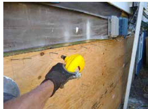
Cripple walls are sheathed with plywood fastened in a tight nailing pattern.
