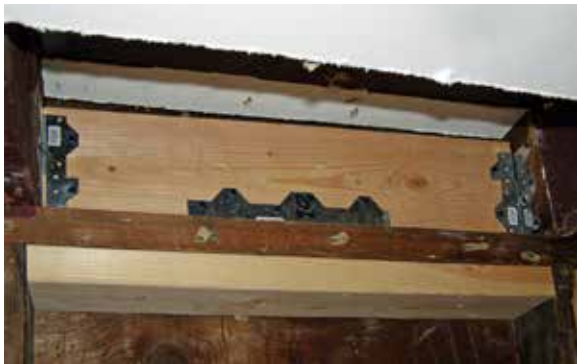
Shear transfer ties connect the top of the cripple wall to the joists above and the floor diaphragm to the top plate.
