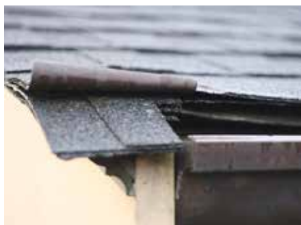
Fig. 7 Metal rain diverter directs water into gutter
