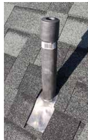
Fig. 4 Lead plumbing stack flashing
