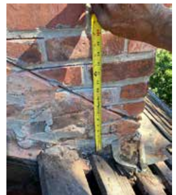
Fig. 3 If previous counter-flashing was set into a diagonal groove cut into bricks, this must be repaired with colour-matched mortar.
