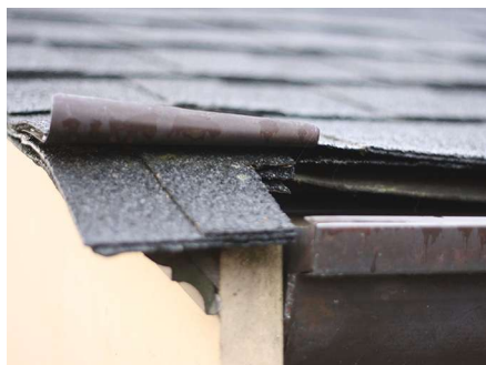
Fig. 7 Metal rain diverter directs water into gutter
