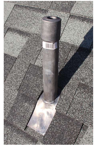
Fig. 4 Lead plumbing stack flashing
